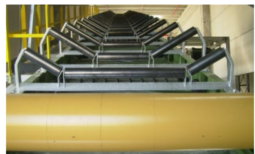
FIGURE 68: THROUGH CONVEYOR FRAME
